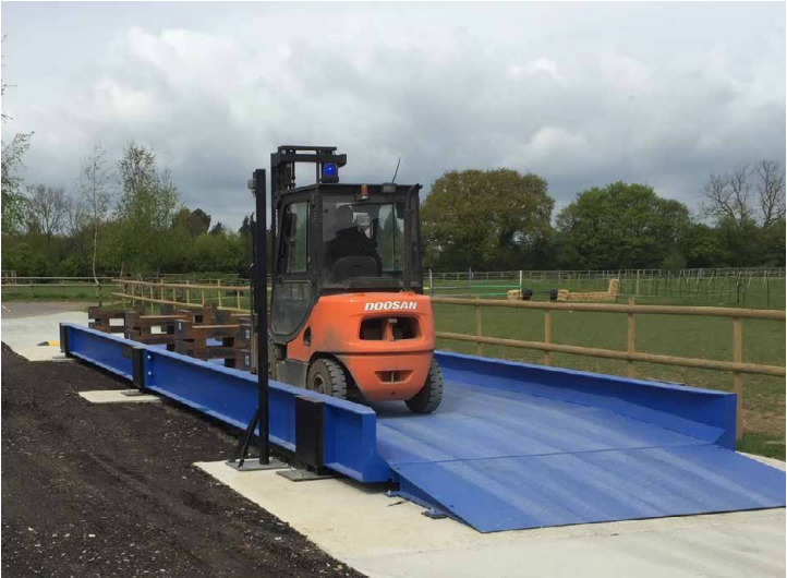
Project: Full turnkey installation including foundations at AWM Potatoes, March Weighbridge: Weighbridge Services 15m x 3m Drive Through with integral 1.5m ramps.
