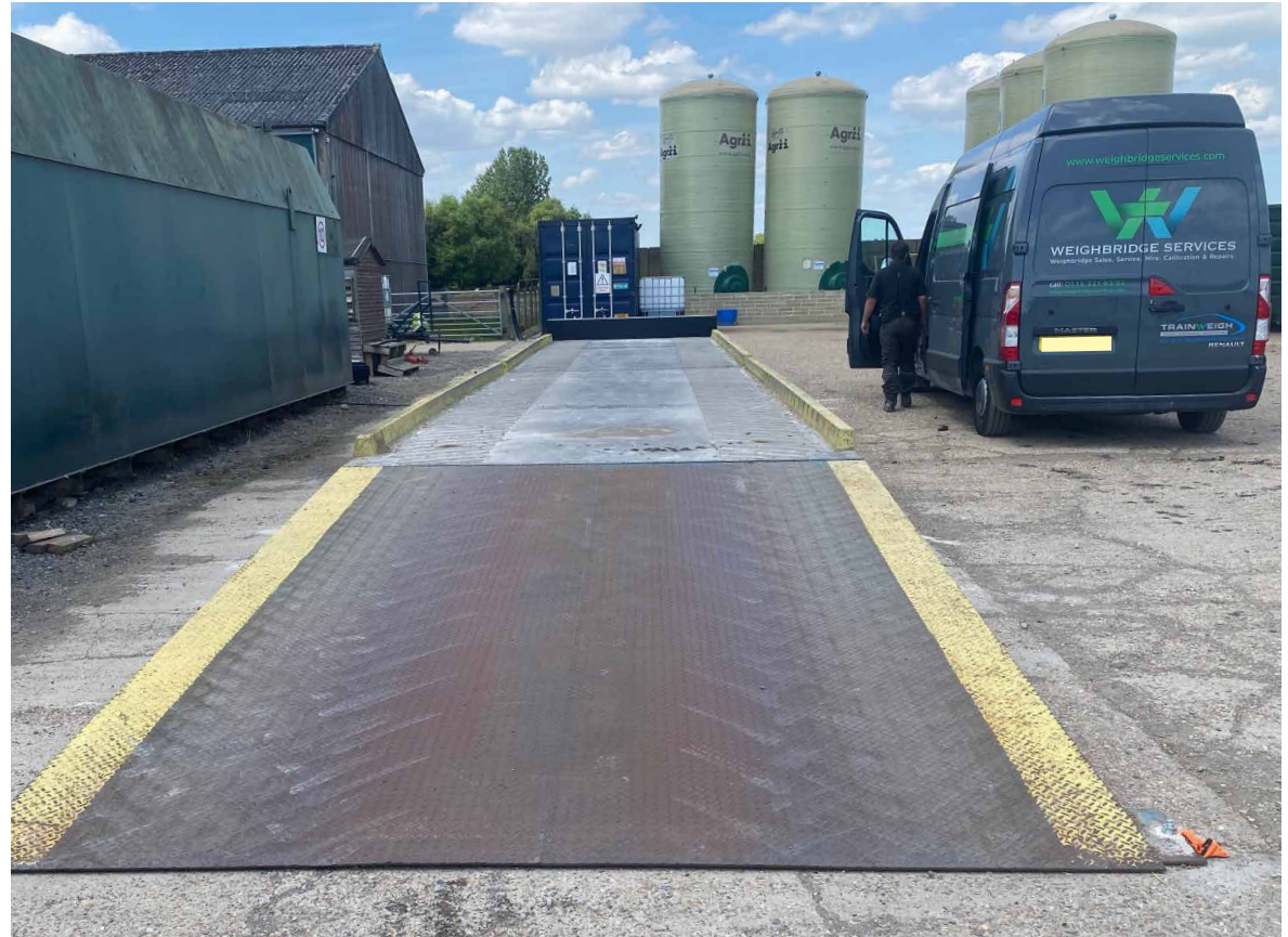
Project: Hire Weighbridge installation at A A Clifton in Bromney Marsh Weighbridge: 15m x 3m concrete weighbridge with ramp and end stop
