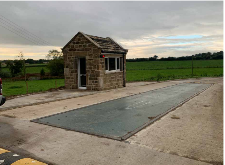
Project: Full turnkey installation including foundations at J E Dickinson, Ardsley Weighbridge: Weighbridge Services 18m x 3m pit mounted.
