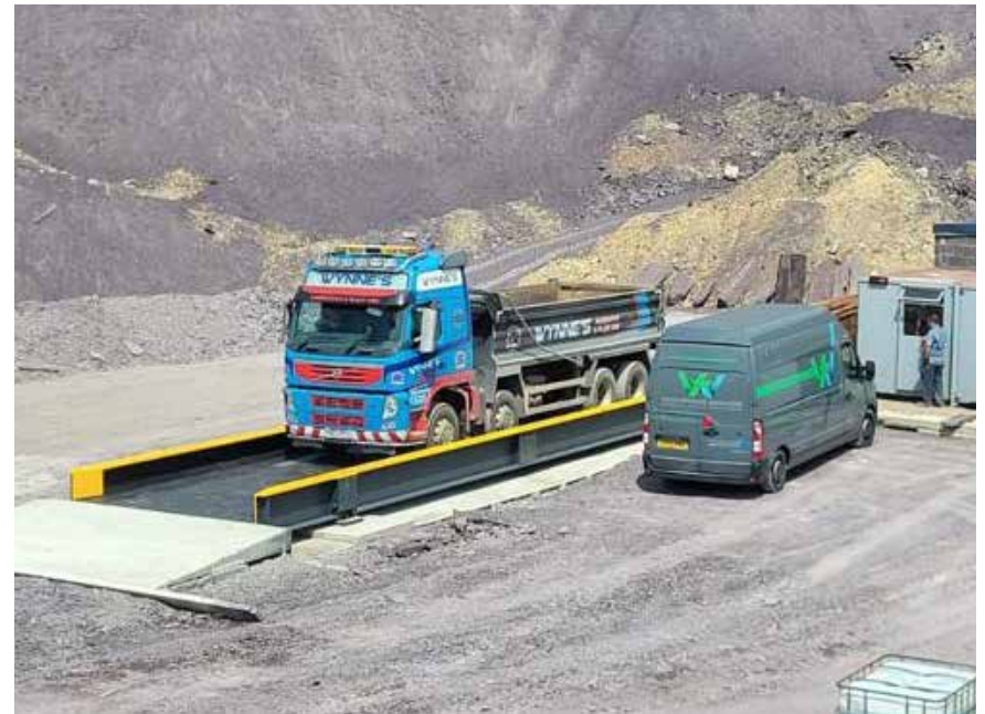
Project: Full turnkey installation including foundations at Celtic Quarries, Bakewell Weighbridge: 15m x 3m Drive Through with concrete ramps
