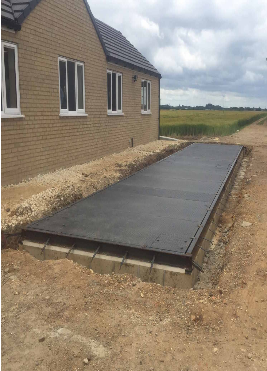
Project: Full turnkey installation including foundations at Linwood Crops, March Weighbridge: 18m x 3m pit mounted.
