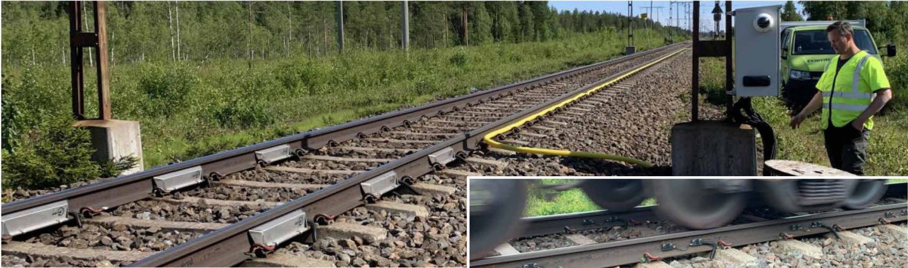
Picture 1 WIM fully installed (with sensor protection shields).
